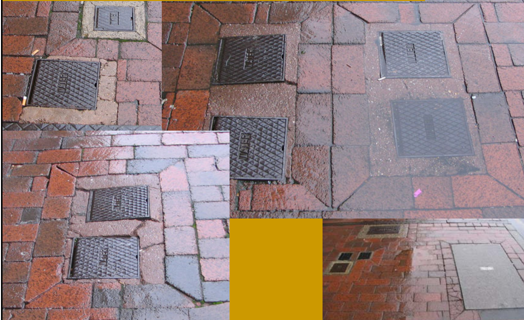
Pavement – brick pavement patched with tarmac or concrete
