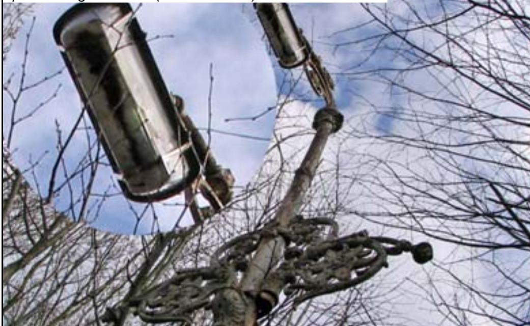
Lamp post with Heritage value in need of restoration
