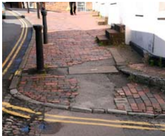
Poor quality footpath on Market Street
