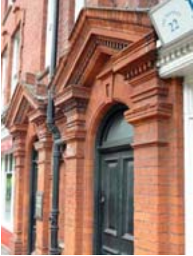
Building decay on London Road
